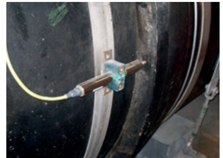
Each spigot and bell socket is monitored using sensors
