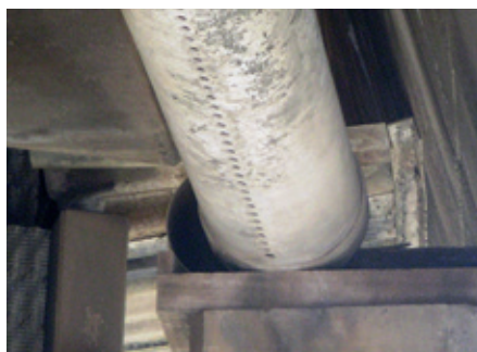
Status survey: Pipes slipped off the fittings due to incorrect installation
